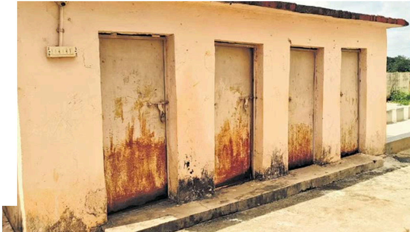
The washrooms that are closed in the Tribal Welfare Residential School in Bommareddygudem, Choutkur mandal, Sangareddy district. Photo | Express
